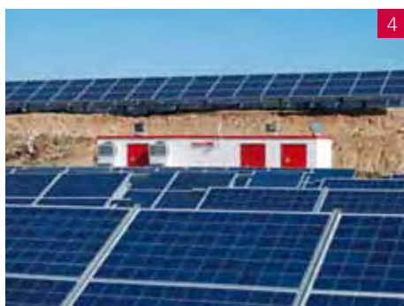
4. CANTIERI ITALIANI Concrete housing at Sardegna (Italy) 9 MW (10 INGECON® SUN PowerMax)
